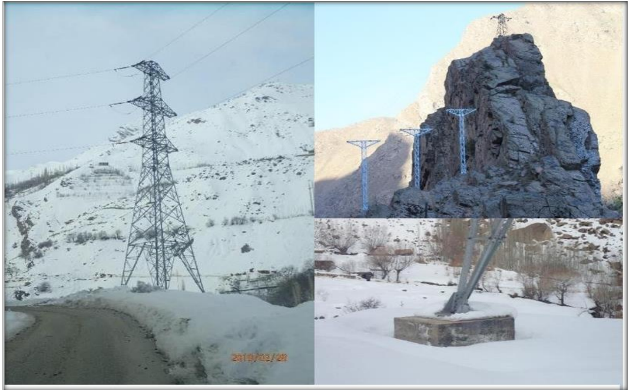
Figure 9 Examples of towers: angle tower at left, three suspension poles on uneven terrain at upper right, and example of foundation at lower right
