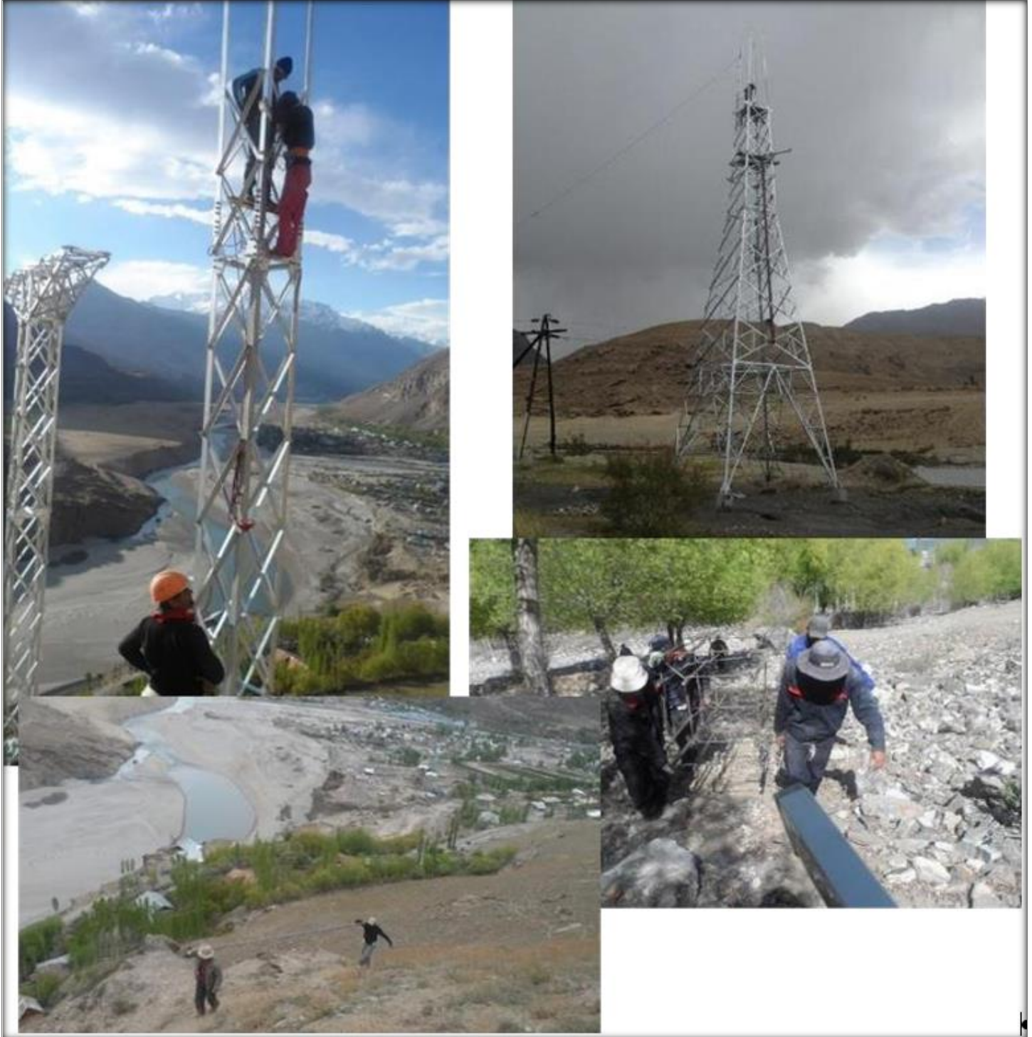
Figure 10 Tower construction process will not use mechanized equipment other than hand tools. The partly assembled tower at top right shows its modular nature, which facilitates hand transport. (source: Pamir Energy)
